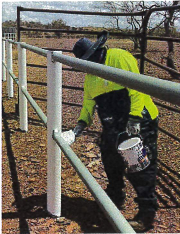
Yinhawangka ranger, Allissa Limerick painting recently completed fence work around a burial site on Rocklea Station.
